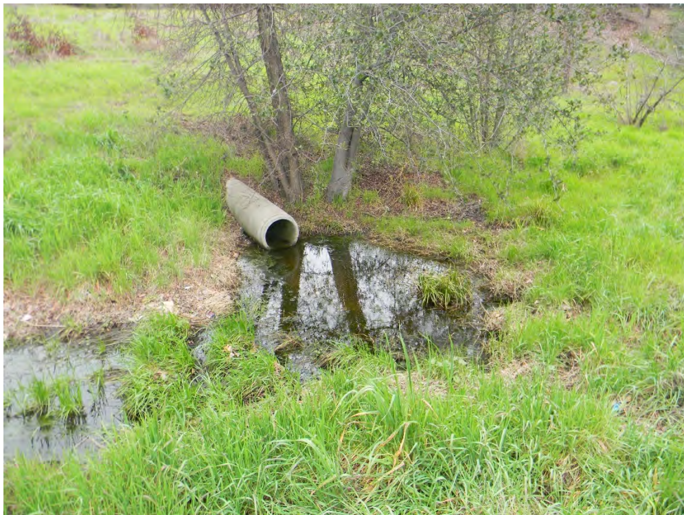
6. Southeastern part of site, view to northeast showing culvert outfall along smaller of two intermittent streams.
